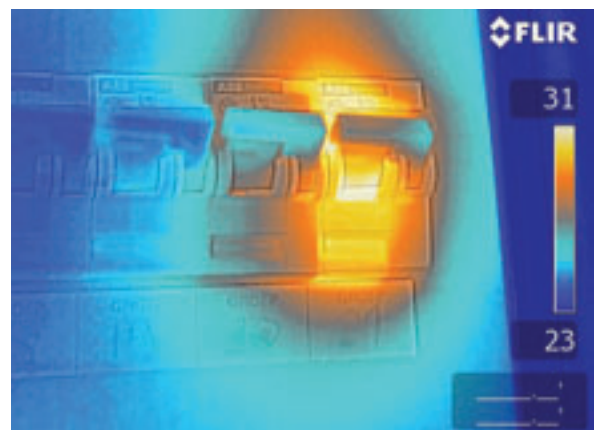
Thermal image of the same overheated fuse, now using the MSX-setting. Note that the text below the fuse is readable, making it very easy to identify and repair the correct fuse at a later stage.
